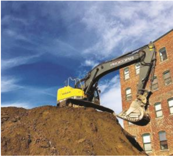
An excavator working on Procopio Cos.’ 259-unit, 10-story tower in downtown Lynn works atop a pile of dirt on the construction site in mid-2018. Photo courtesy of Procopio Cos.
