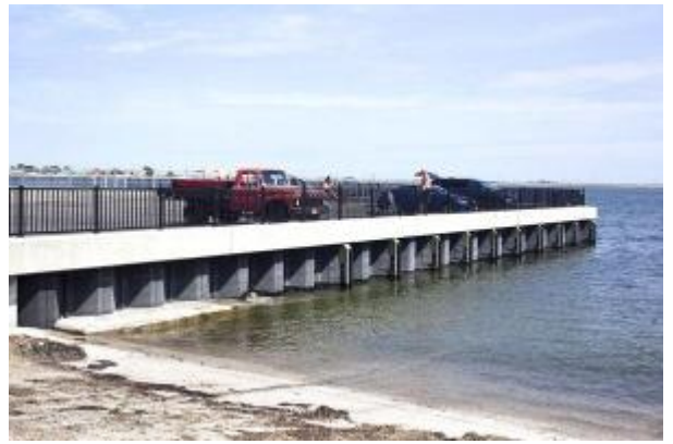
The Blossom Street extension, which will be the ferry terminal, shows progress on Friday as one of several projects on the Lynn waterfront. (Item Photo / Angela Owens)
