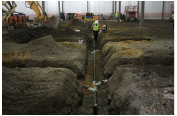
Workmen install drains in what will be the production area of the new Kettle Cuisine Company located next to the Clock Tower building in Lynn.
